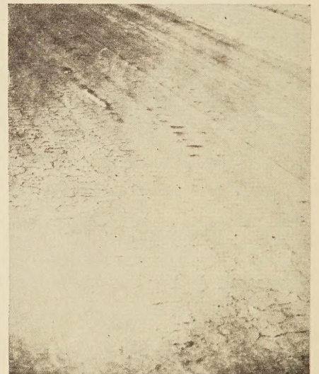
SURFACE PITTED AND CHECKED
